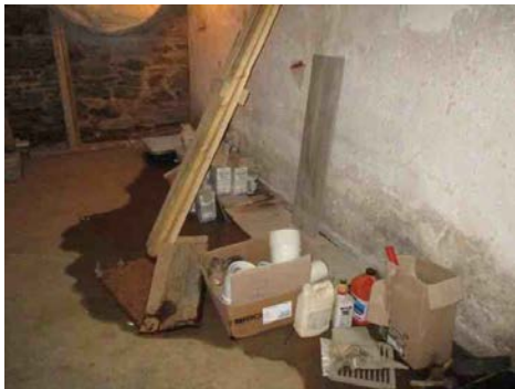
Basement (Stndng Wtr)
