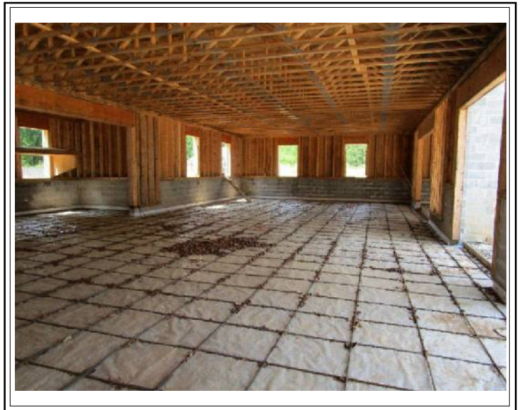
5/Car Detached Garage - Interior
