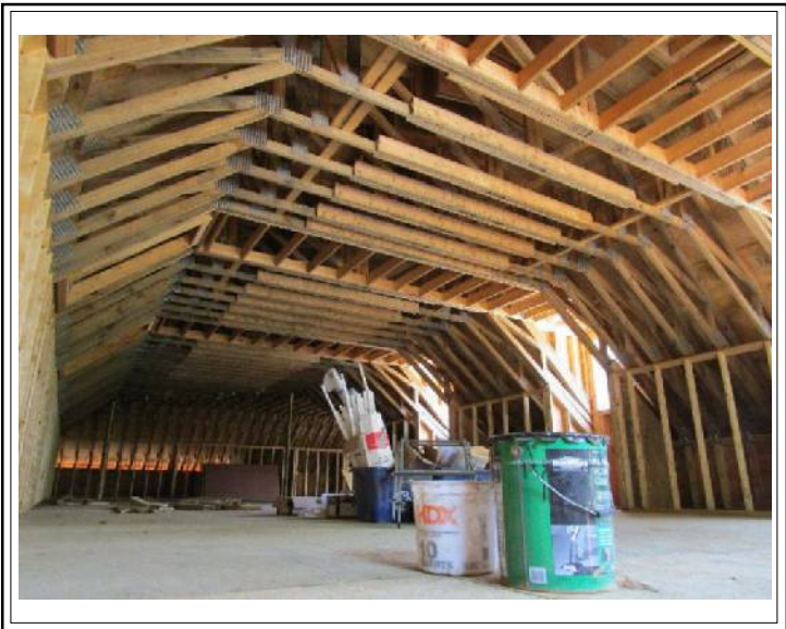
5/Car Detached Garage - Interior
